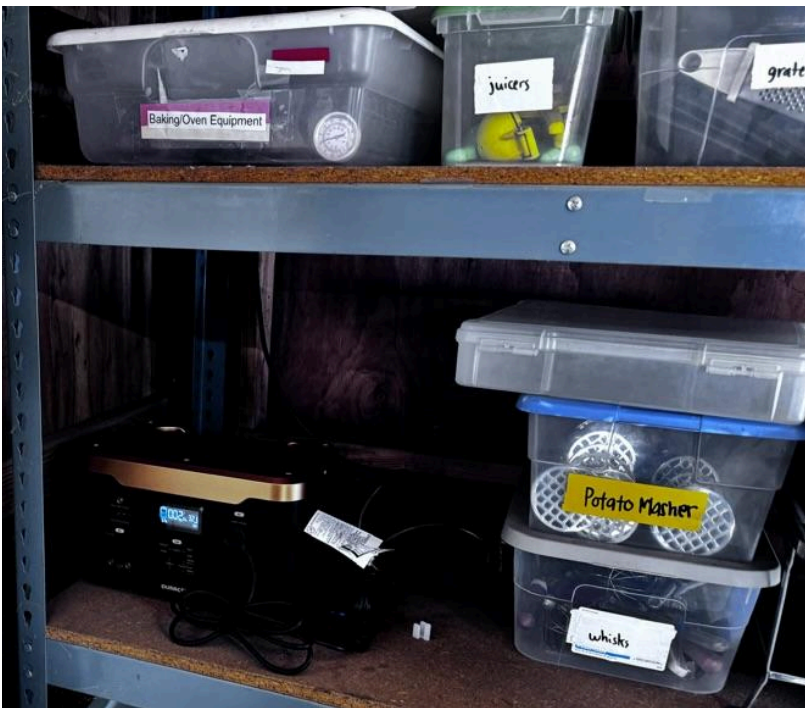
Figure 4. Solar Battery In Use on Cocina Shelf
