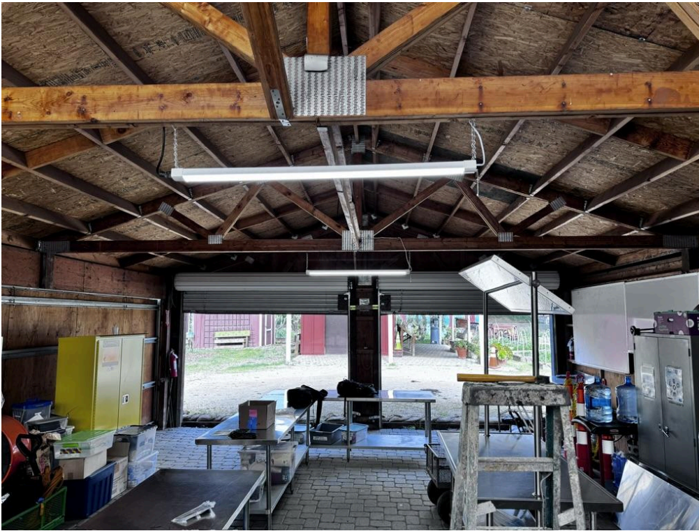
Figure 3. Cocina with Installed and Connected Lights
